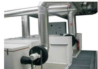
Vehicle Air Conditioning Test Chamber
